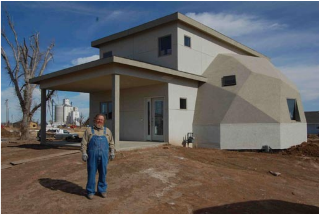
Scott Eller is building a home of "SIPs," or structurally insulated panels.
